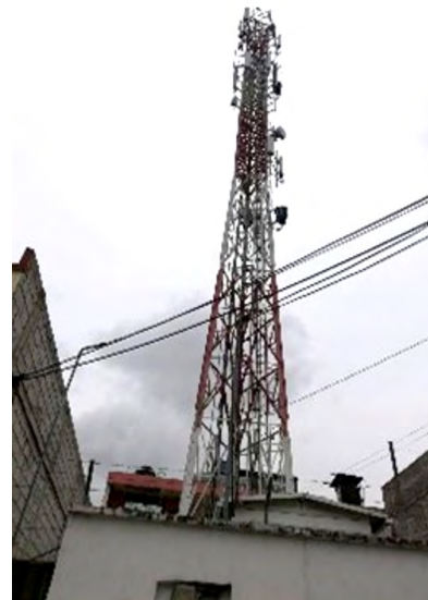
Fig. 4. Figure 4 Base Station
